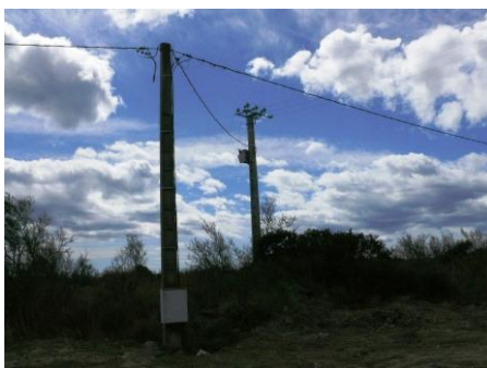
Part of the electric lines
